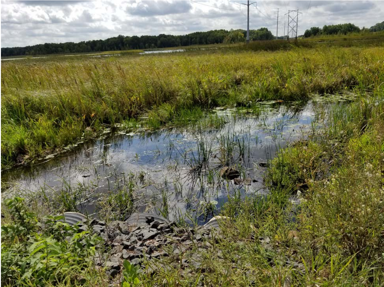
Photo: outlet pipes from Swamp Lake
