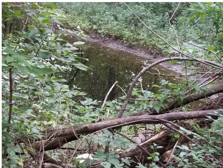
Photos: Right – Downed trees at Sportsman Drive culvert
