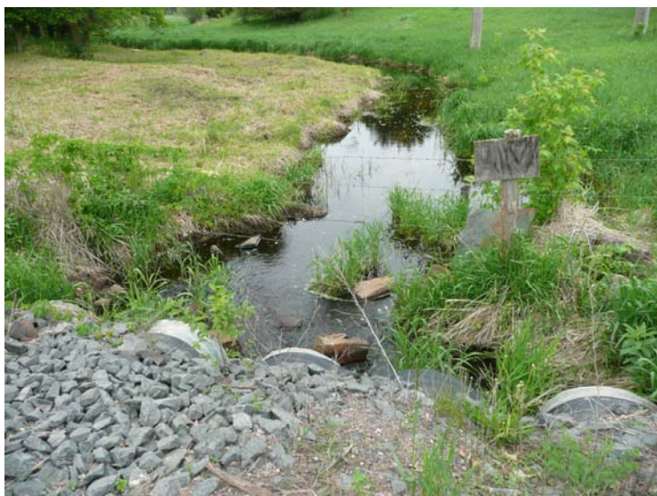
Photos: Pipes leaving Swamp Lake
