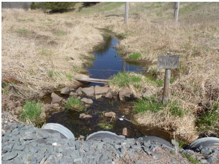
Photos: Pipes leaving Swamp Lake
