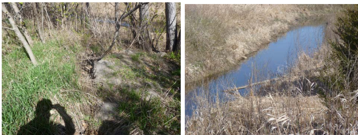
Photos: Left: Erosion cause by flow from adjacent farm field, Right: Downed Tree in Channel
