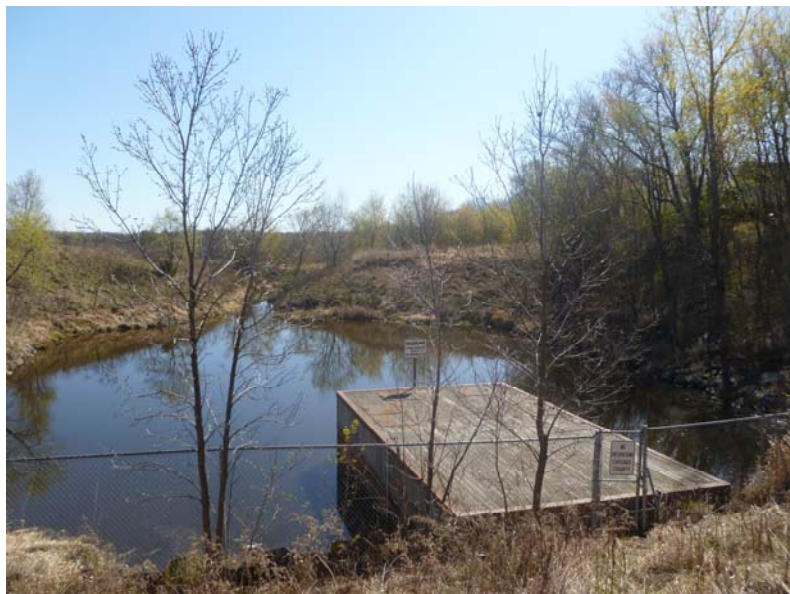
Photos: Outlet structure from Chisago to Green
